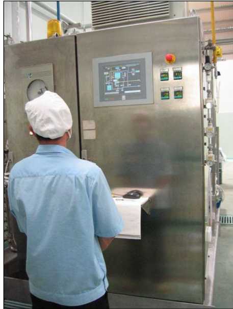
Electric Board with PLC
